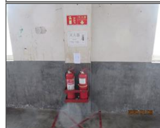
External photo(s) of the production unit(s) fire extinguishers.JPG
