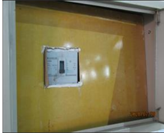
External photo(s) of the production unit(s) 7.13 corrected_the electric box with insulation protective equipment.JPG
