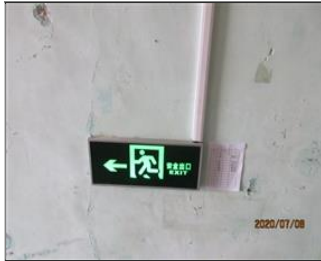
External photo(s) of the production unit(s) evacuation exit sign.JPG
